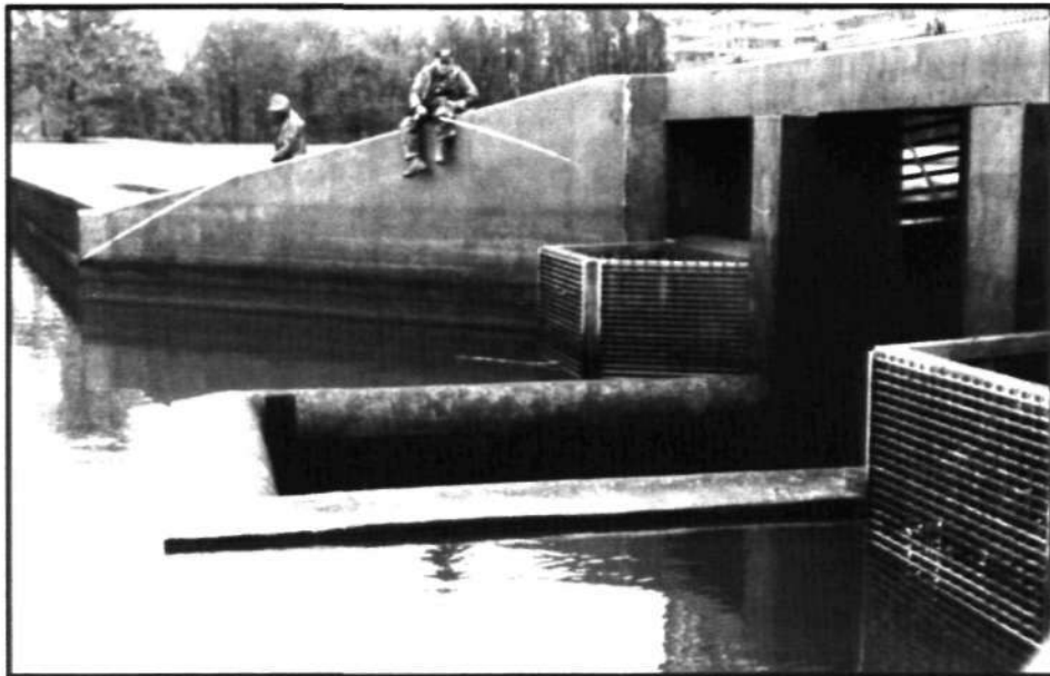
Figure 4. Upstream view of dam highlighting spillway and fish screens above sluice gates
