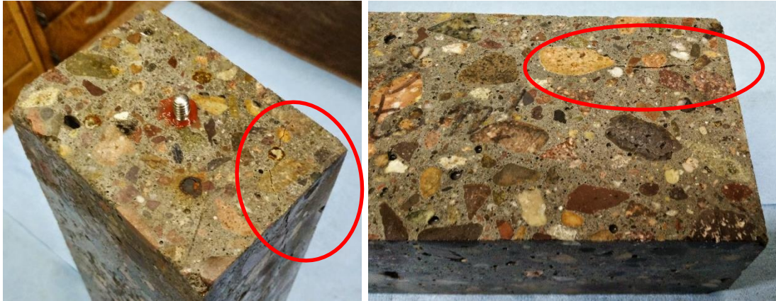
Figure 1-1 Example of artificial damage of excised beam from concrete crosstie for ASTM C666 testing. Circles point to extensive cracking due to saw-cutting (from Riding et al. , 2016).
