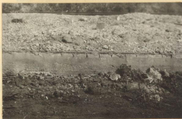
Second coat of grout applied too thick
