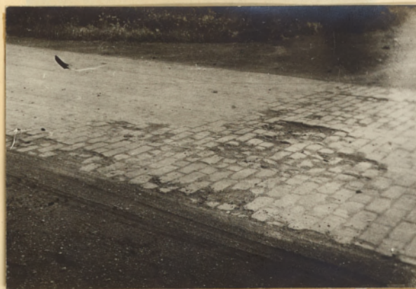
Typical expansion joint failure
