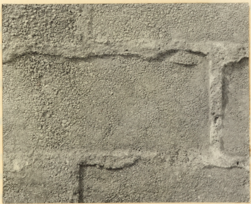
Close view of separated base, showing effect of laying wet brick on dry mix
