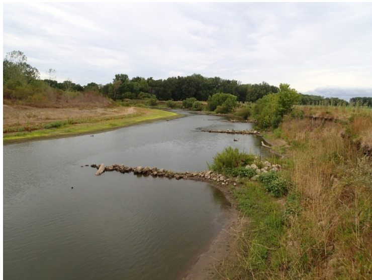
Figure 16: Bank erosion with lower bank protection at Mackinaw River
