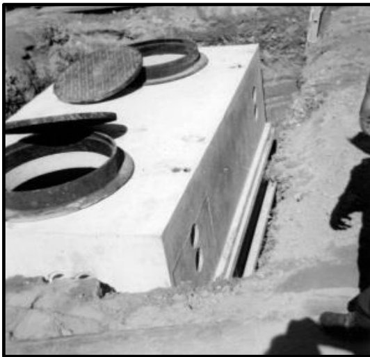
Figure 15. The top shell of the facility being lowered into place, ca. summer 1971.
