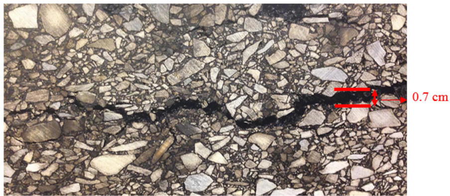
Figure 5.6: The presence of the large cracks in the asphalt concrete
