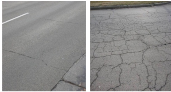
Figure 1.2: Thermal cracking (left) and block cracking (right) on asphalt concrete pavements in Illinois.
