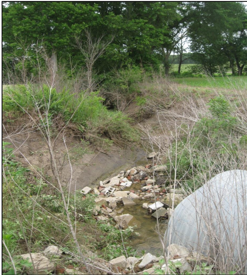
Figure 4. Vegetation cleared and in-channel culvert installed at Site 3. Looking downstream (Photo by Alex W. Peimer).
