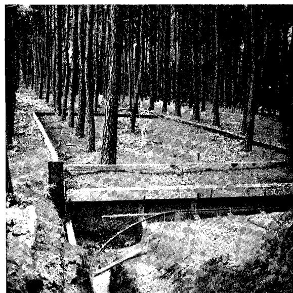
Fig. 22. Plot No. 1 ready for operation.
