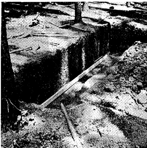
Fig. 15. Access pit at the lower end of Plot No. 1. Note the black vinyl already laid in the side trench.
