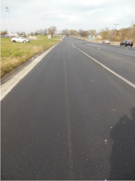
Figure 19. Segment 2 (between I-57 and I-80). Slightly cracked surface in center of photo defines edge of level binder and cold-milling taper to curb line.
