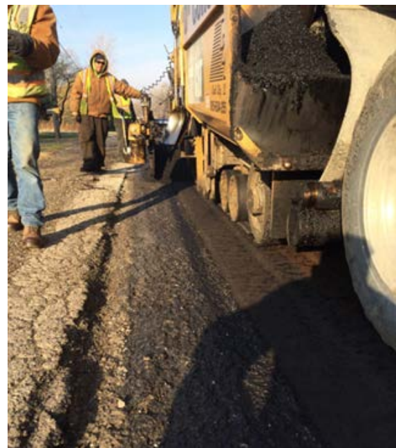
Figure 26. Surface course installation showing leveling course, lip between level and cold-milled surface, and surface course installation.
