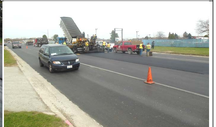
Figure 18. Segment 2 (between I-57 and I-80). Placing surface course installation on Pulaski. Primary straight section with cold-milling from curb to 6 ft from curb. A 24-ft longitudinal grade reference was used in lieu of the 30 ft required.
