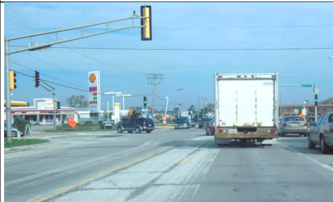
Figure 13. Segment 2 (between I-57 and I-80) cold-milled pavement.
