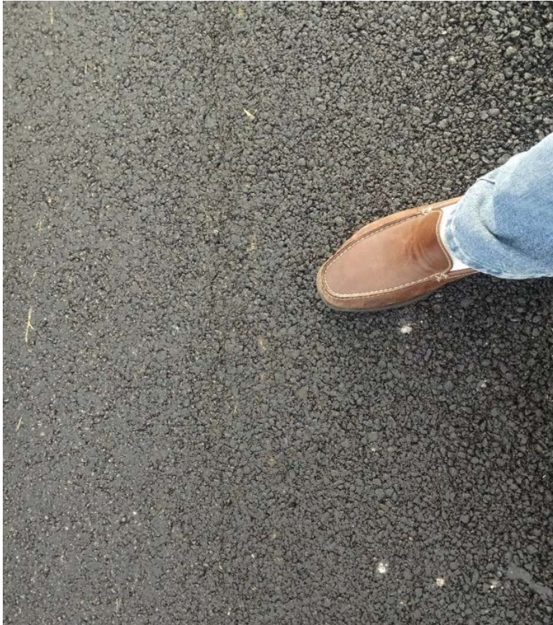
Figure 27. Evidence of hairline crack at underlying transition from level binder to no level binder. Level binder (4.75 mm) to left of crack and milled surface to right of crack. Increased segregation also at pavement edge (right side of photo).
