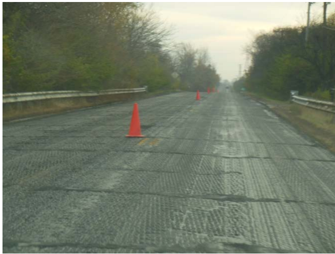
Figure 23. In Segment 2, the milling resulted in loss of material at numerous cracks and joints that had reflected through the previous HMA overlay.
