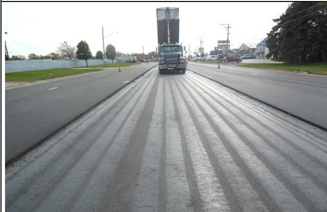
Figure 17. Segment 2 (between I-57 and I-80). Placing surface in turn lane. Typical zebra-striped tack coat on level binder.
