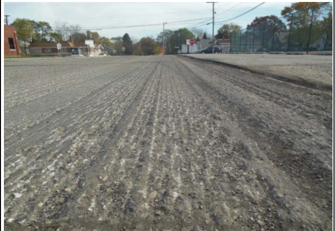
Figure 22. Existing cold-milling specifications do not address variability between adjacent teeth; newer teeth result in deep grooves of 0.5 in or more across the pavement section (Segment 1 shown).
