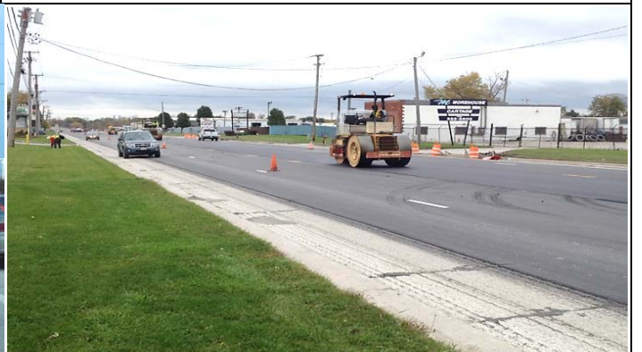
Figure 14. Segment 2 (between I-57 and I-80) level binder placed at start of cold-milled taper.
