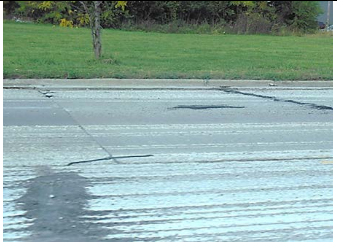
Figure 10. Segment 2 (between I-57 and I-80) cold-milled pavement.
