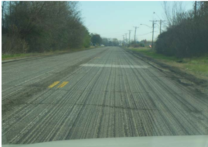
Figure 21. Segment 2 cold-milling of roadway exposed numerous previously installed pavement patches.
