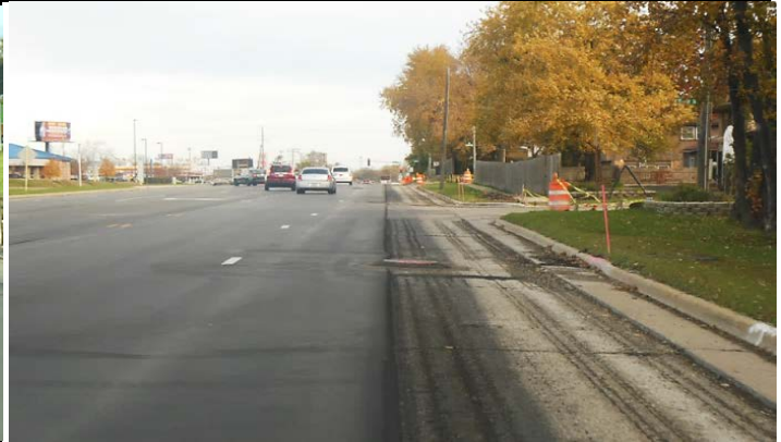
Figure 16. Segment 2 (between I-57 and I-80). Placing 4.75-mm level binder course from approximately 6 ft off of curb line. Level binder course is 1 in thick at 6 ft off of curb line, not tapered to zero.
