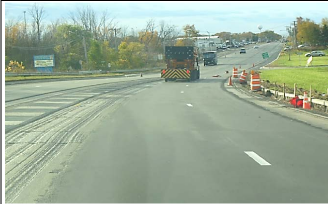
Figure 15. Segment 2 (between I-57 and I-80). Placing 4.75-mm level course from approximately 6 ft off of curb line and 6 ft from center median.
