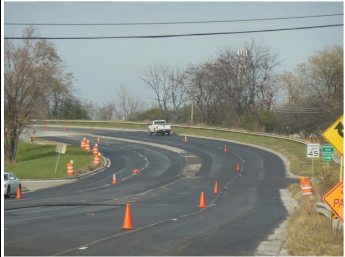
Figure 20. Segment 2 (between I-57 and I-80). Slightly cracked surface (lighter surface area) defines location of level binder. Right 6 ft of lane (darker area next to curb) is cold-milling taper where the surface is 2.5 in at center of lane tapering to 1.5 in at curb.
