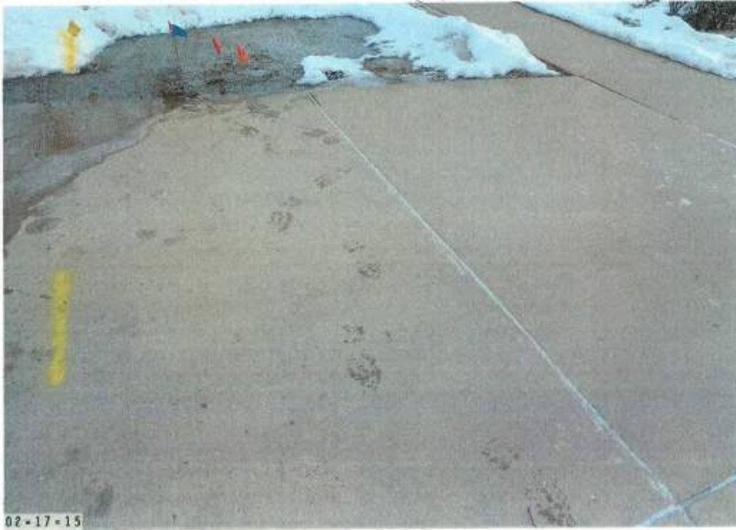
Figure B.1 Sample photos taken by staff at locations of leaks.
