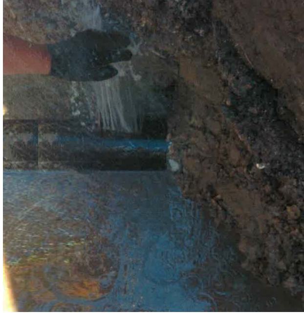
Figure 3.4 Leak on a six inch pipe Kincaid Court.
