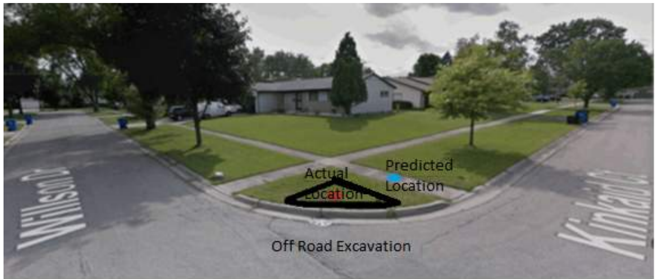
Figure 3.3 Location of hidden leak showing predicted location (blue) versus actual leak location (red).
