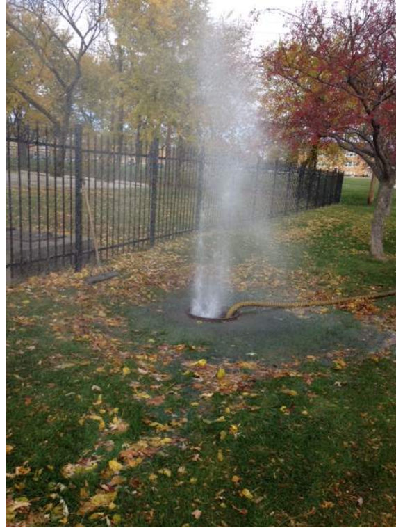
Figure 3.5 Linneman Road leak in meter pit on shutoff valve.
