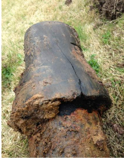
Figure 1.4 Cracked pipe from Liberty, PA. Leak found by acoustics.
