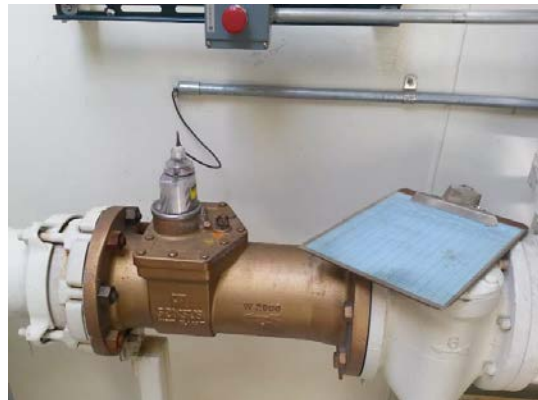
Figure 2.4 Master meter tracking flow into system from adjoining utility interconnection.
