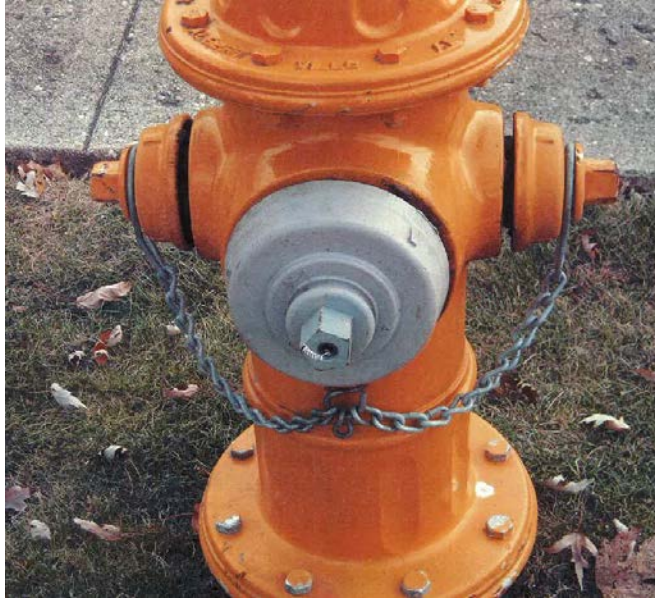
Figure 4.1 Damage on hydrant cap.
