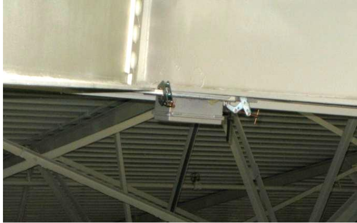
Figure 7.5 Imote2 sensor node attached to the center truss.
