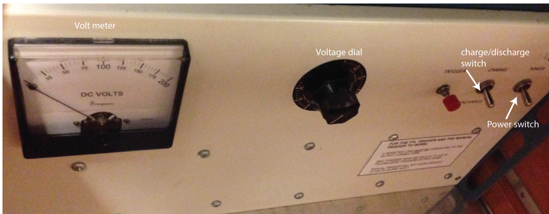
Figure 25 Capacitor bank control panel with key controls labeled.
