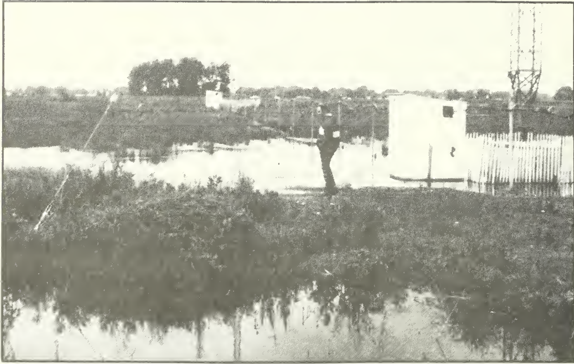
Figure 13. Water forming a pond in a sag subsidence.
