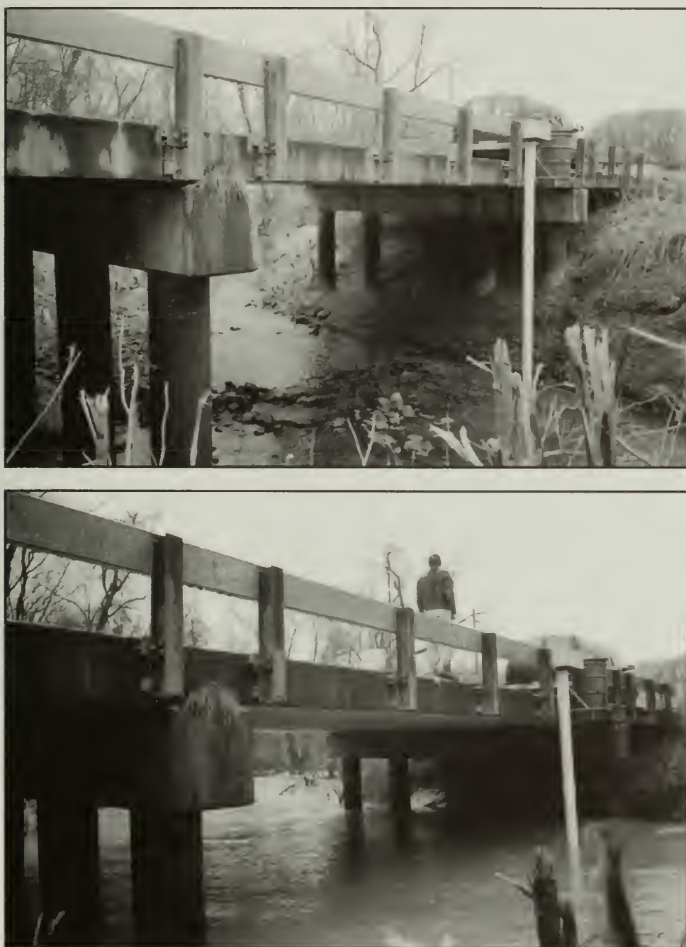
Figure 2 The bridge monitoring site at base flow (top) and flood stage (bottom). The box, pipe, and 55-gal drum mounted to the side of the bridge (on the right) contain a data logger, electrodes, and an ISCO automatic water sampler, respectively.
