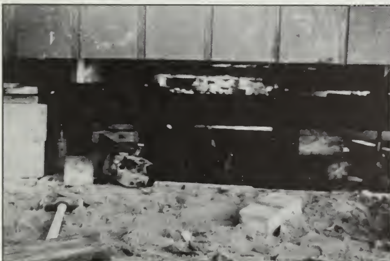
Figure 11 (above) Concrete blocks of a crawl space have been removed to make room to jack the house to a level position. (below) A closer view of the crawl space shows the I-beams supporting the releveled house.
