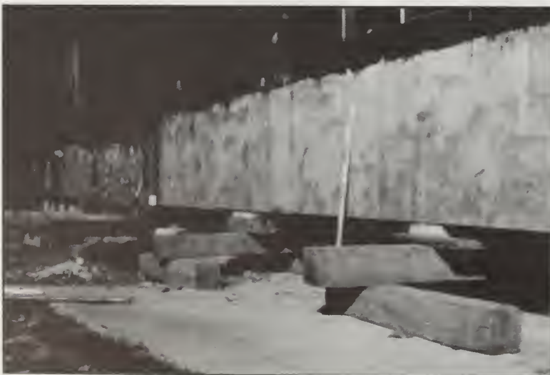
Figure 10 Bearing walls of a house on a slab. The entire superstructure has been jacked up to a level position, exposing the interior.
