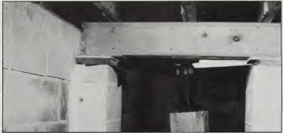
Figure 14 Main beam is not attached to the foundation. Because of differential settling, cracks develop in the house above the beam.
