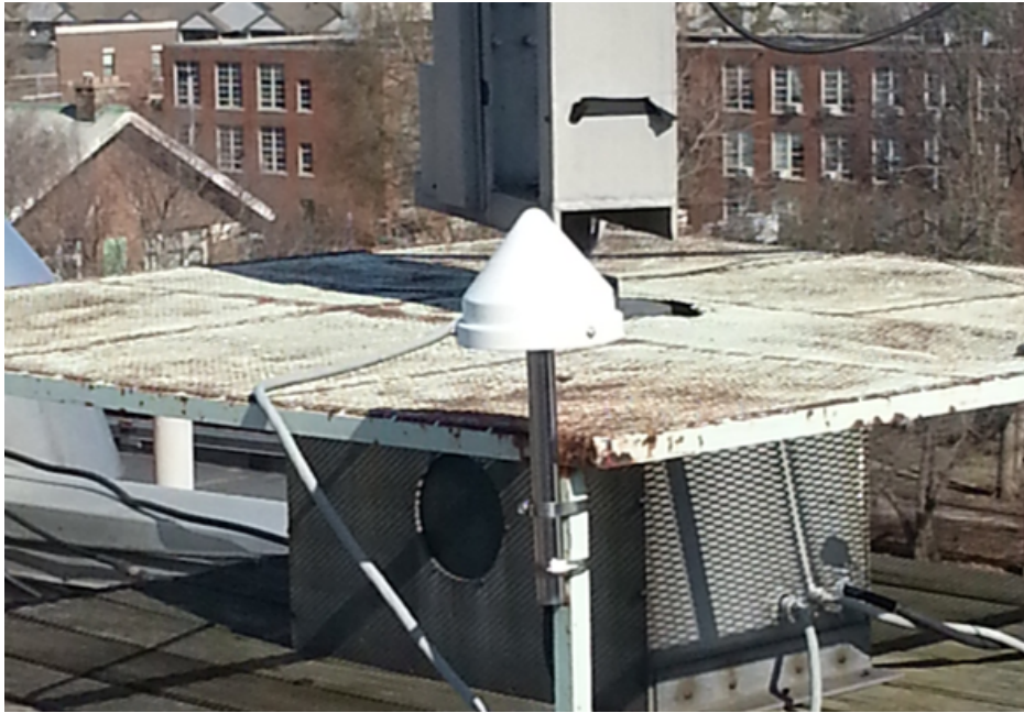
Figure 3.6: Fixed reference antenna with full access to the open sky.
