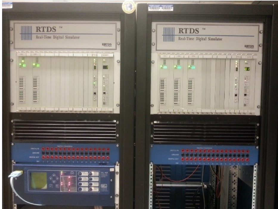
Figure 2.3: A real-time digital simulator of power systems at the University of Illinois at Urbana-Champaign. The RTDS is capable of simulating large-scale power systems in order to test the effects of disturbances on the power grid.
