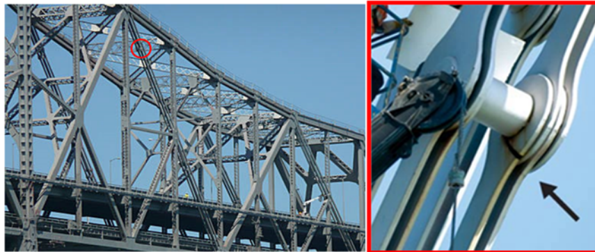
Figure 0.10. San Francisco-Oakland Bay Bridge and cracked eye bar by fatigue.
