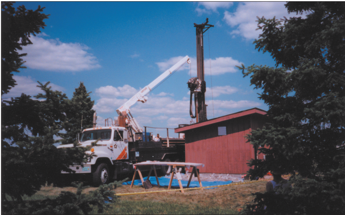
Figure 6 Drilling operations with rotasonic drill rig immediately adjacent to the well house for NIWC 57. Core recovery was almost 100%, and drilling fluids were not used.
