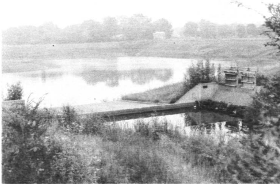
Figure 13. In-channel flood retention basin and inlet control spillway on Addison Creek between miles 9.75 and 10.00
