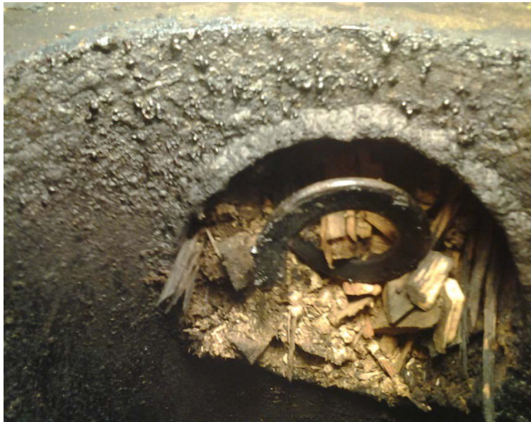
Figure 13. The auger exit at the top of the gasifier. The auger was clogged due to large pieces of wood chips.
