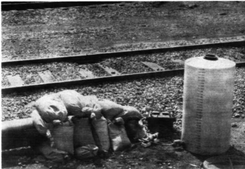
Figure 7. Dye tank and metering pump
