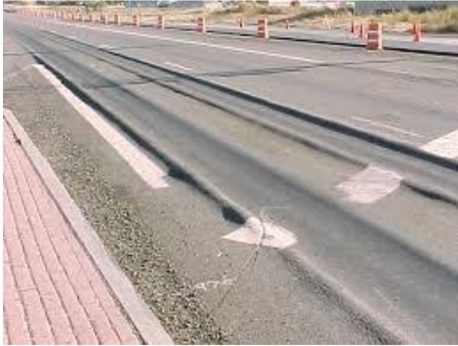
Figure 0-6: Rutted Road Surface Occurs with Too Soft Asphalt Binders (Gotame, 2016).
