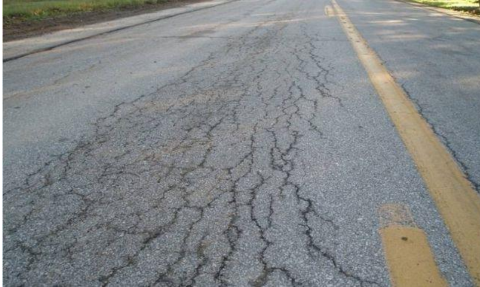
Figure 0-7: Fatigue Cracked Road Surface Due to too Hard Asphalt Binders Being Used (Galal and White, 2001).
