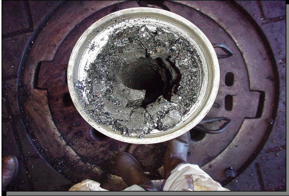
Figure 0-4: An Asphaltene Deposit Formed on the Inside of a Pipeline in a Refinery (Mckenna, 2009).
