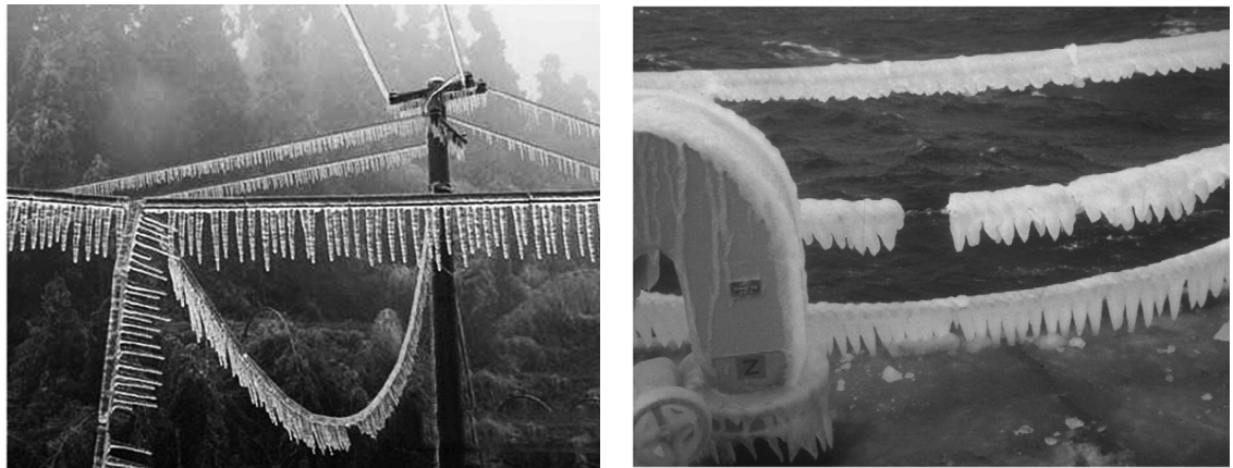
Figure 1.2. Ice accumulation on transmission lines [1], [15]
