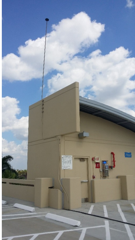
Figure 7. The antenna on the stairwell creating interference.
