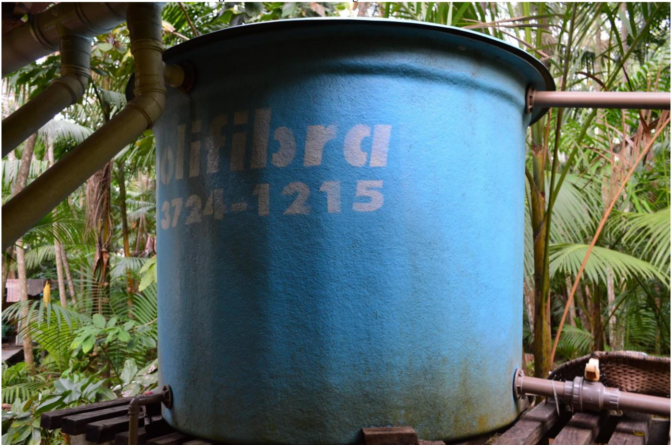
Figure 2. Rainwater harvesting installation on Jutuba
