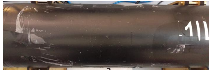
Fig. 11. Pipe sample with saltwater sealed inside defects (before aluminum foil is applied).
