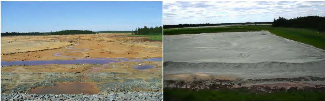
Figure 5.1 Manitou TSF 2 site before (June 2008) and after (August 2012) the installation of a 1.2 to 2.1 m thick cover made of non-acid-generating tailings from Goldex mine.
