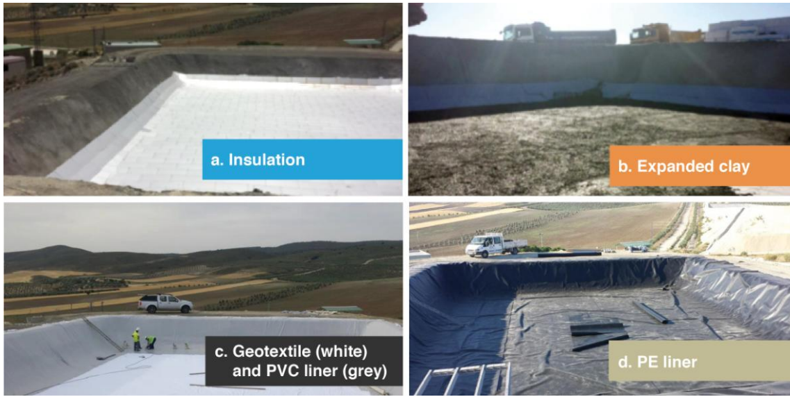
4 Figure 1. Insulation and lining of the Granada solar pond: details of installation of materials and 5 final configuration.
