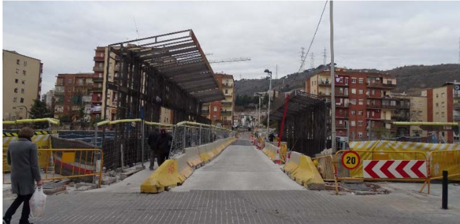
Figure 29. Photograph of the load increase on the non-instrumented span of the bridge taken in January 2016
