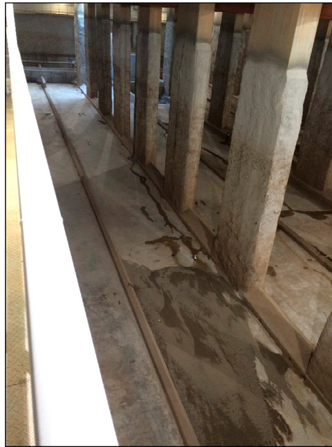
Figure 2. Inside picture of the Estrella storm tank in Badalona and the studied lane.
