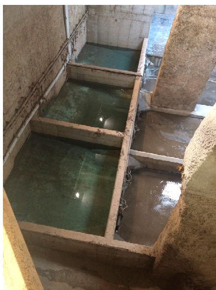
Figure 1. Storage chambers of the Estrella storm tank with a flushing gate cleaning system.
