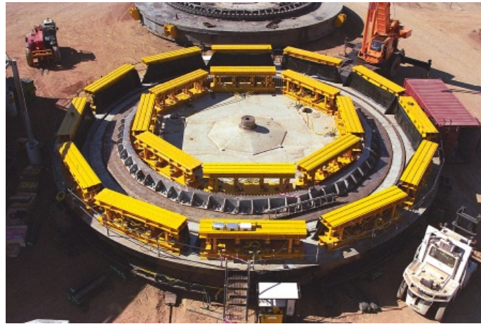
Figure 92. Synchronous hydraulic lifting system to lift a 3500 tons mining dragline in Australia. Engineered by Enerpac.
