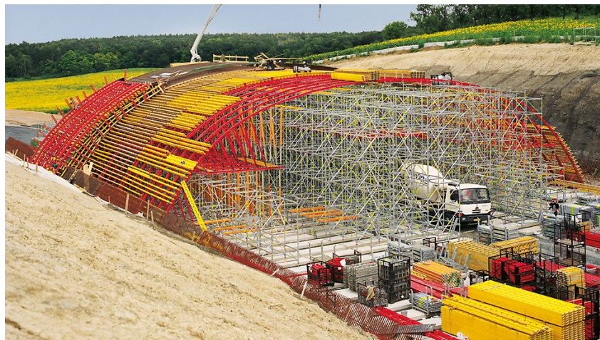
Figure 80. Open-cut tunnelling method. Zehun Bridge, Czech Republic. Technology by Peri. Source: https://www.peri.com/en/projects/civil-engineering/deer-crossing-bridge-zehun.html
