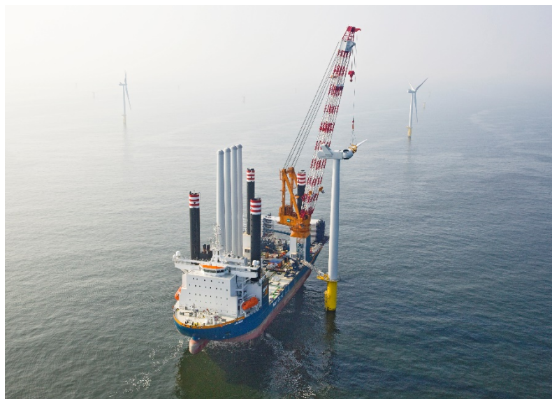
Figure 30. Brand-new installation vessel Aeolus started its first job at the Eneco Luchterduinen Source: http://www.offshorewindindustry.com .
