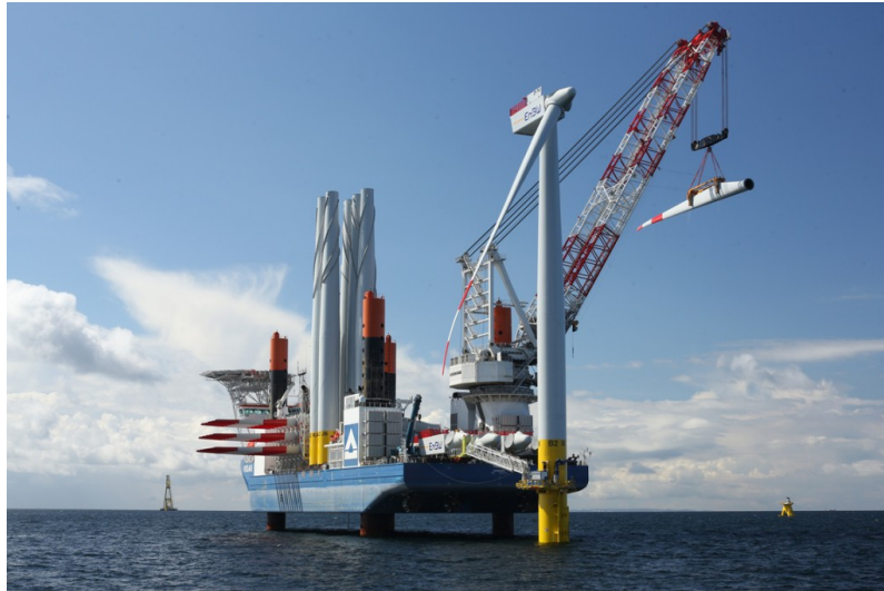
Figure 29. Hochtief jack-up vessel Vidar during lifting operation of second blade. Source: http://www.offshorewindindustry.com/news/jan-de-nul-acquires-jack-vessel-vidar
