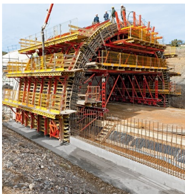
Figure 68. Exterior tunnel falsework with working decks used in road construction of RN 88, France. Technology by Peri.
