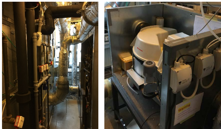
Figure 5.2.3. Prototype of the air cleaner installed in the ventilation system is shown with a section of the air handling unit.
