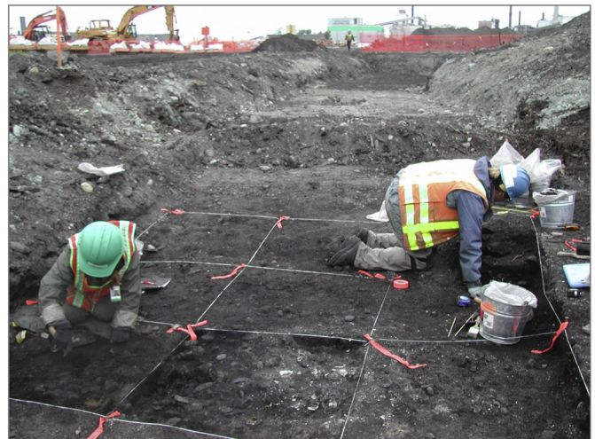
Fig. 4. Photograph showing archaeological excavation (foreground) in the dry dock project construction zone. Note the depth of fill between the modern ground surface (indicated by heavy machinery) and the pre-industrial, 19th century surface where field technicians Rene Casebeer (left) and Kim Kwarsick (right) are excavating. Photo #248, taken on May 25, 2004 by Sarah Sterling. Used with permission by Washington State Department of Transportation and the Burke Museum of Natural History and Culture.
