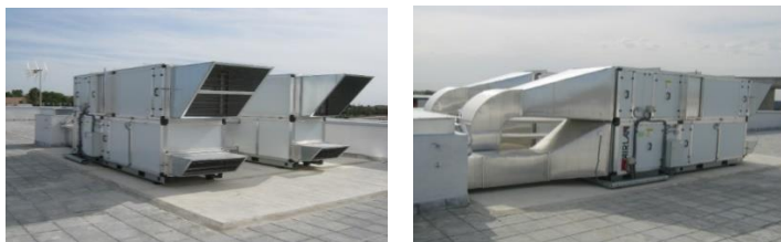
Fig. 4. Mechanical Ventilation system in an Andalusian school. Roof tops.
