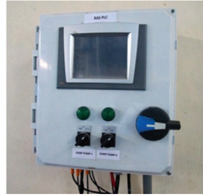
Programmable Logic Controller of the RAS
