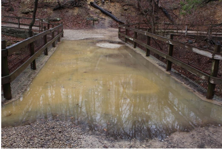
Figure 12: This is an extreme example of flooding on a bridge. The bridge had no drainage system installed, thus, stopping water from dispersing.
