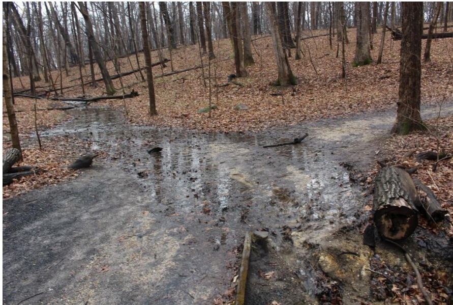
Figure 13: This is an example of a flooded pathway. This pathway became flooded due to a lack of drainage.
