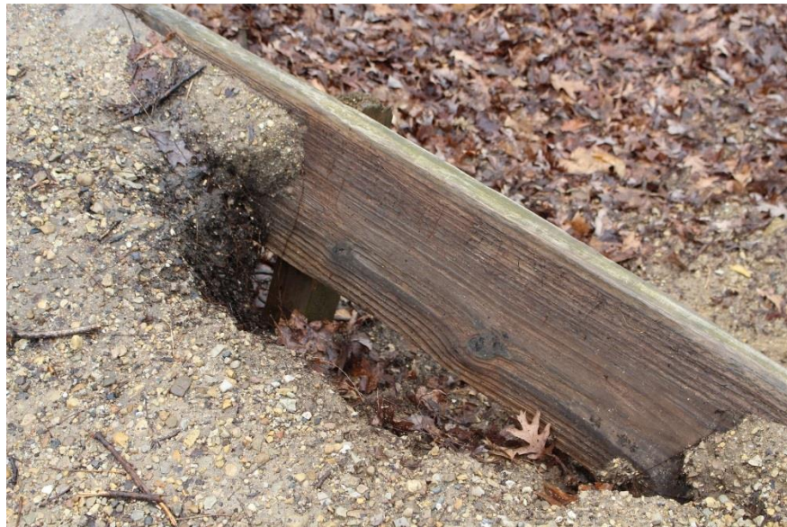
Figure 15: This photo shows how the support structure is failing as the water has removed the soil and a hole has developed.
