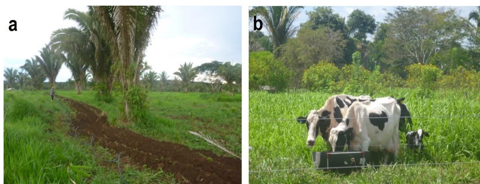
Figure 9. (a) Installation of underground piping to deliver water to each plot in the Silvopastoral System with Rotational Grazing for Dairy initiative; (b) Dairy cattle drinking from one of the water troughs, with electric fencing in the foreground.
