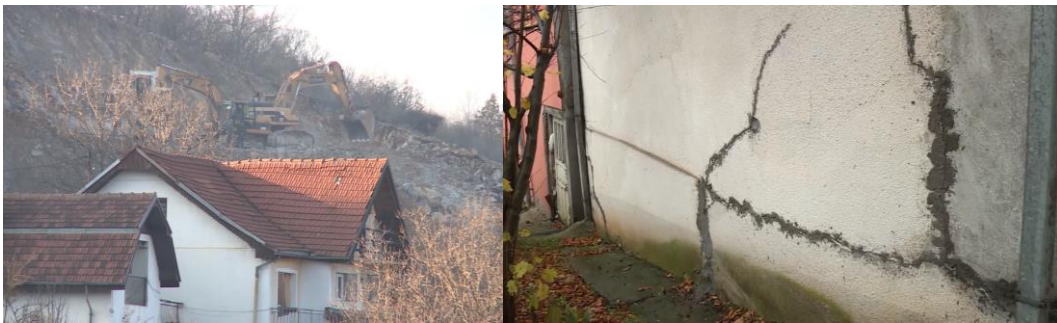
Figure 1. Damages on the houses caused by quarry excavation activities, Resource: http://rs.n1info.com/a210245/Vesti/Vesti/Dimitrovgrad-Mestani-cekaju-odstetu-Koridora.html
