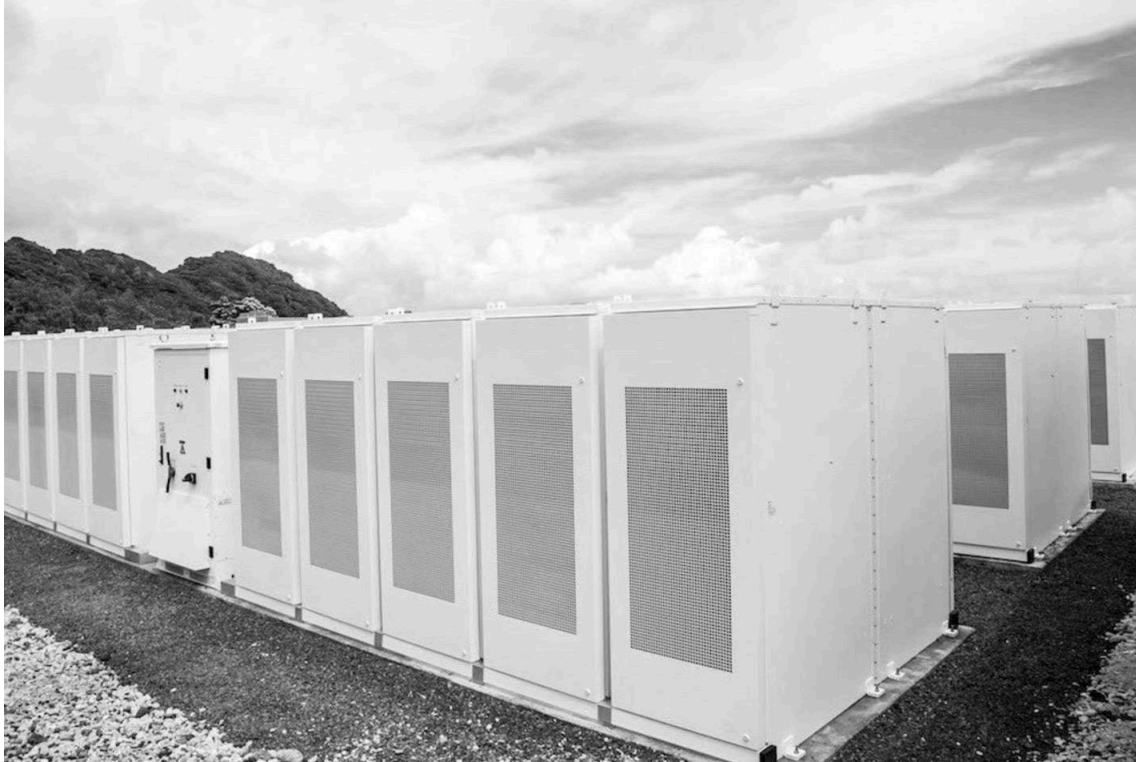
Figure 3.11 – Lithium-ion based Tesla Powerpacks (6 MWh) (SolarCity, 2017).
