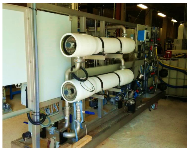
Figure 5.2 – Pressure vessels of the RO unit
