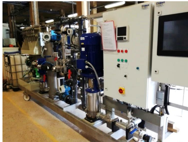
Figure 5.1 – Reverse osmosis unit
