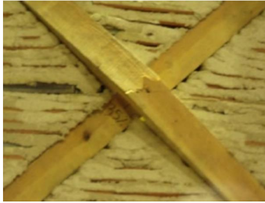
Figure 6.2 - Buckling and rupture of the diagonal - Typical collapse mechanism – Reproduced from (L. Kouris, et al., 2014)
