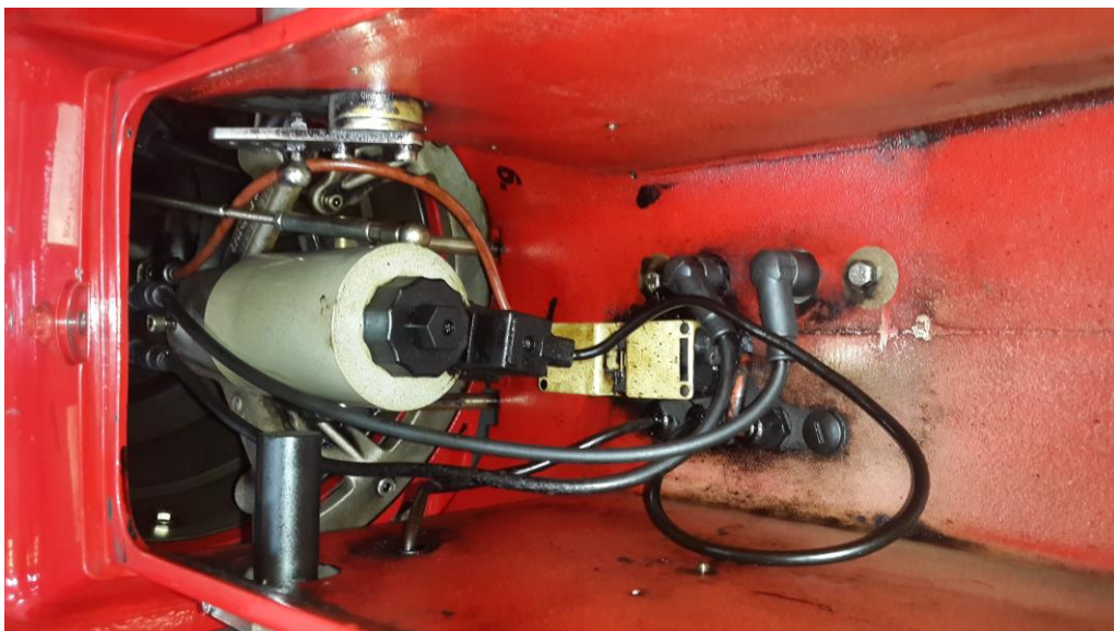
Figure 5.4 Burner mixing head after maintenance work
