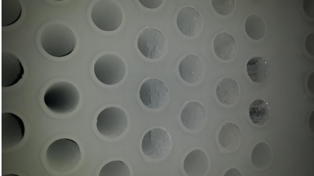
Figure 5.5 Flame tubes without proper maintenance
