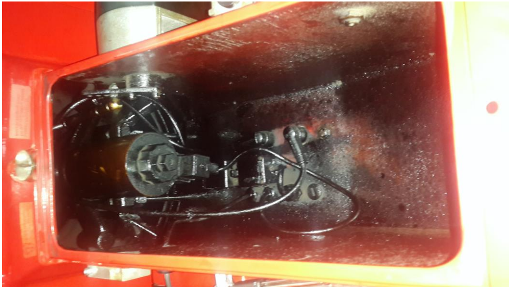
Figure 5.3 Burner mixing head without proper maintenance
