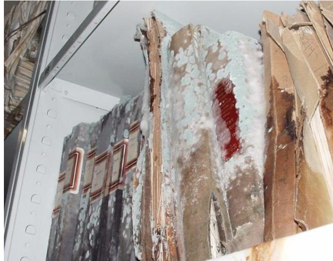
Figure 1.5: Fungal development on archival documents due to water leak in the roof of a depository room. Image courtesy of Arquivo Histórico Ultramarino (AHU-DGLAB, Portugal).
