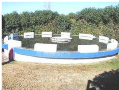
Figure 2.29 Vila Verde WWTP secondary decanter
