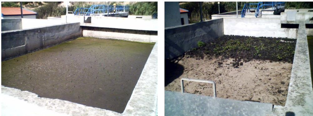
Figure 2.15 Sludge Drying Beds
