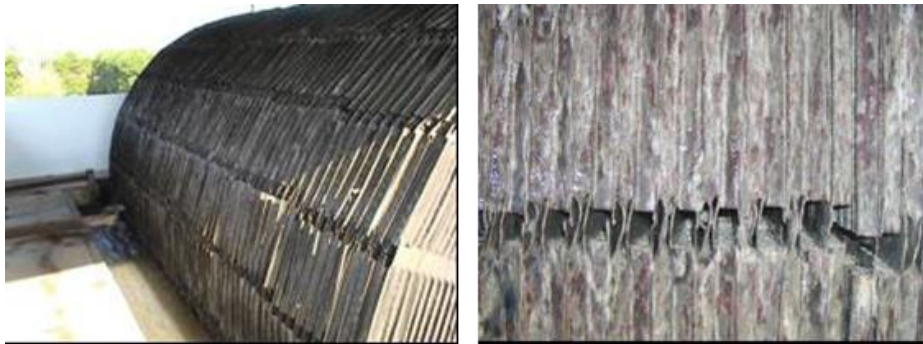
Figure 2.28 Vila Verde WWTP bio-disks
