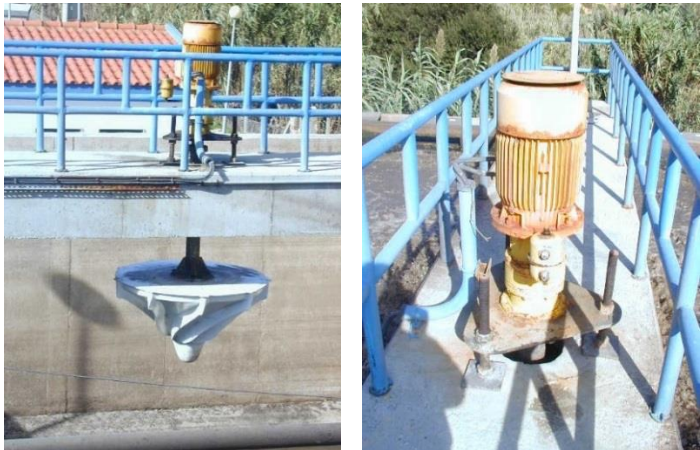
Figure 2.9 Aeration tank turbine.
