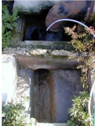
Figure 2.14 Final effluent with sodium hypochlorite injection
