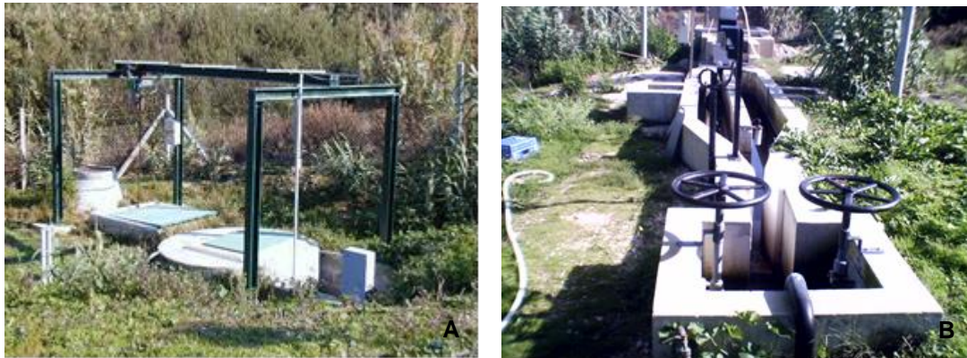
Figure 2.6 A) Affluent entry; B) Parshall channel.
