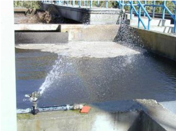
Figure 2.10 Surface spray system.
