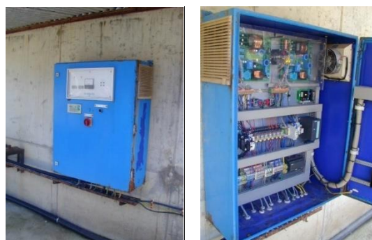
Figure 2.13 Tertiary treatment electric board
