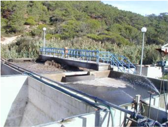
Figure 2.8 Aeration tank and secondary decanter.
