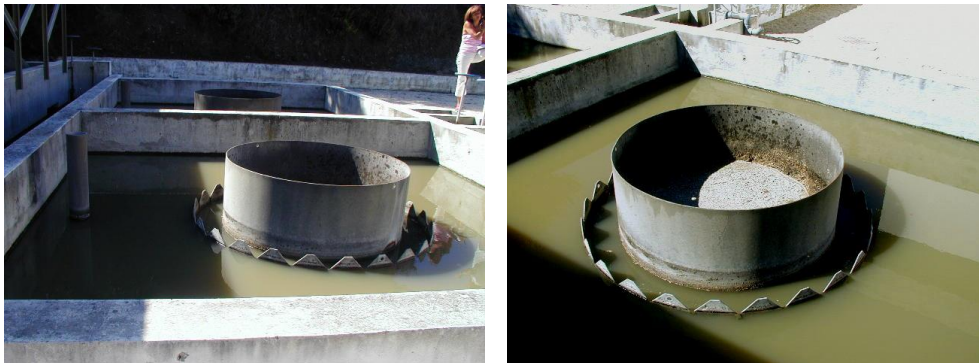
Figure 2.20 Primary sedimentation tanks
