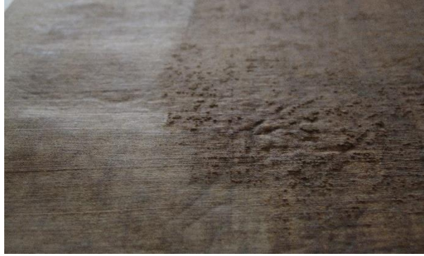
Figure V.15 – Cleaned area on the left (after the lining adhesive was scrapped off) contrasting with the still-uncleaned area on the right side.
