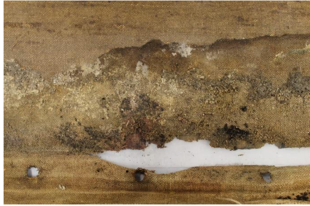
Figure V.7 – Bottom of the lining canvas exhibiting severe disintegration of the material and extensive mould growth.
