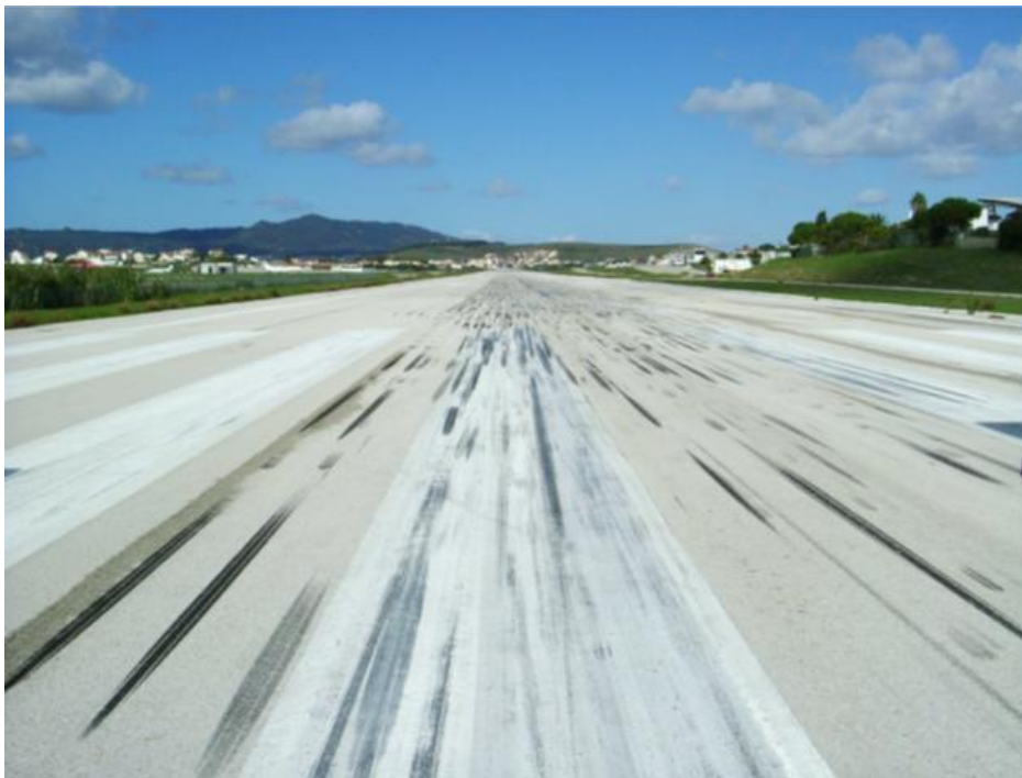
Figure 3.2 - Rubber deposits on the contact area near the threshold 36
