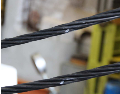
Figure 5.54: Detail of the broken strands
