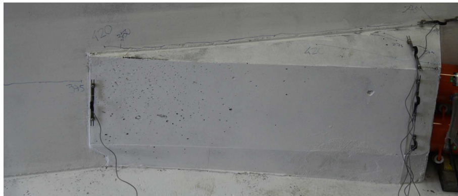
Figure 5.52: Cracking on the anchorage blister
