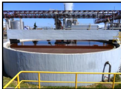
Figure 9 - View of the thickener at Portucel in Setúbal.
