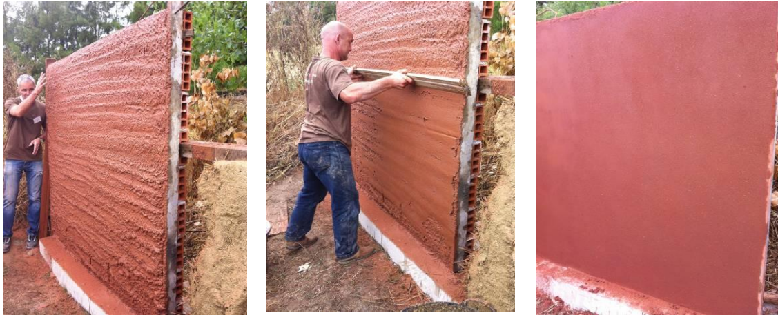
Figure 3. Commercial earth plaster on the hollow brick test wall after projection (left), being levelled (middle) and finished (right)
