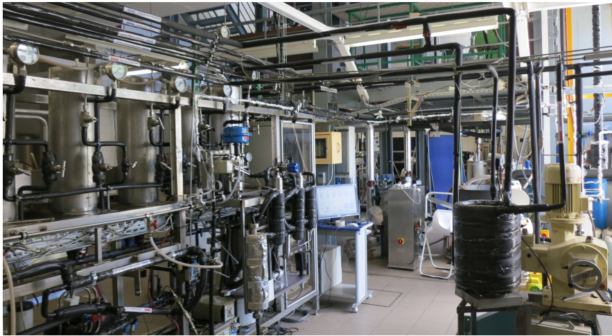
Figure 2.2.2 – High-pressure pilot installation used for continuous biodiesel production.
